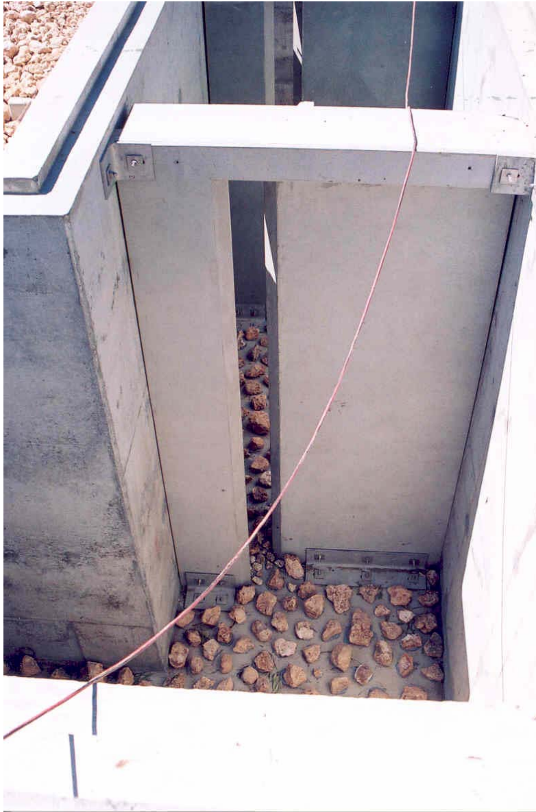
Lock 8 Fishway vertical slot constructed from precast concrete panels, looking upstream. Cobbles have been glued to the floor with epoxy to provide additional roughness, which is intended to assist smaller fish.
