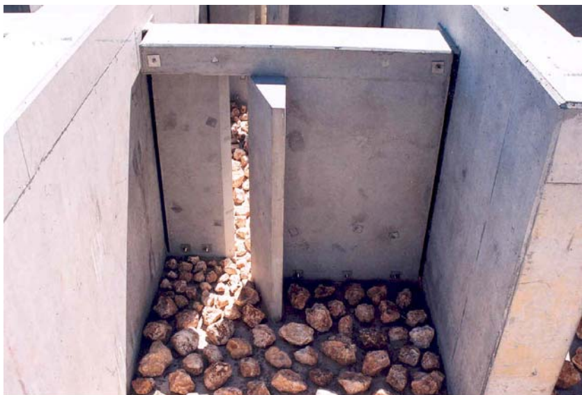
Lock 8 Fishway vertical slot looking downstream.
