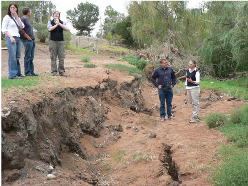
Figure 4. Due to the historically low water levels below Lock 1 and in the Lower Lakes, some of the adjacent land is drying out for the first time in more than 50 years, resulting in cracking and subsidence.
