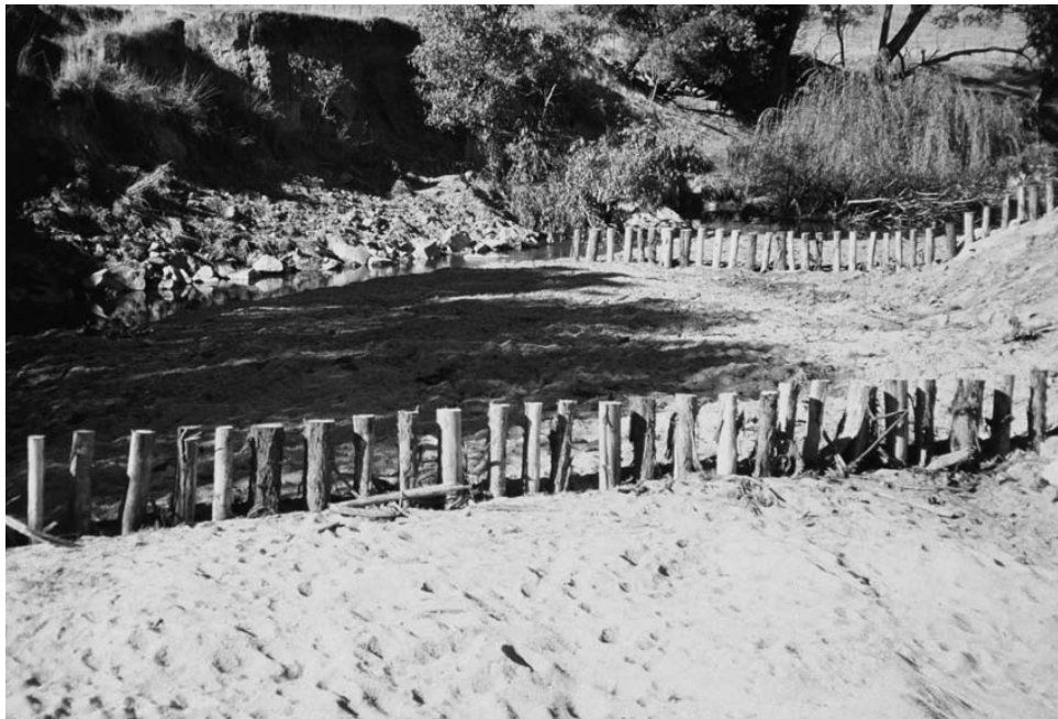
Figure 5. Use of rocks and pile groynes to reduce stream width in Seven Creeks
