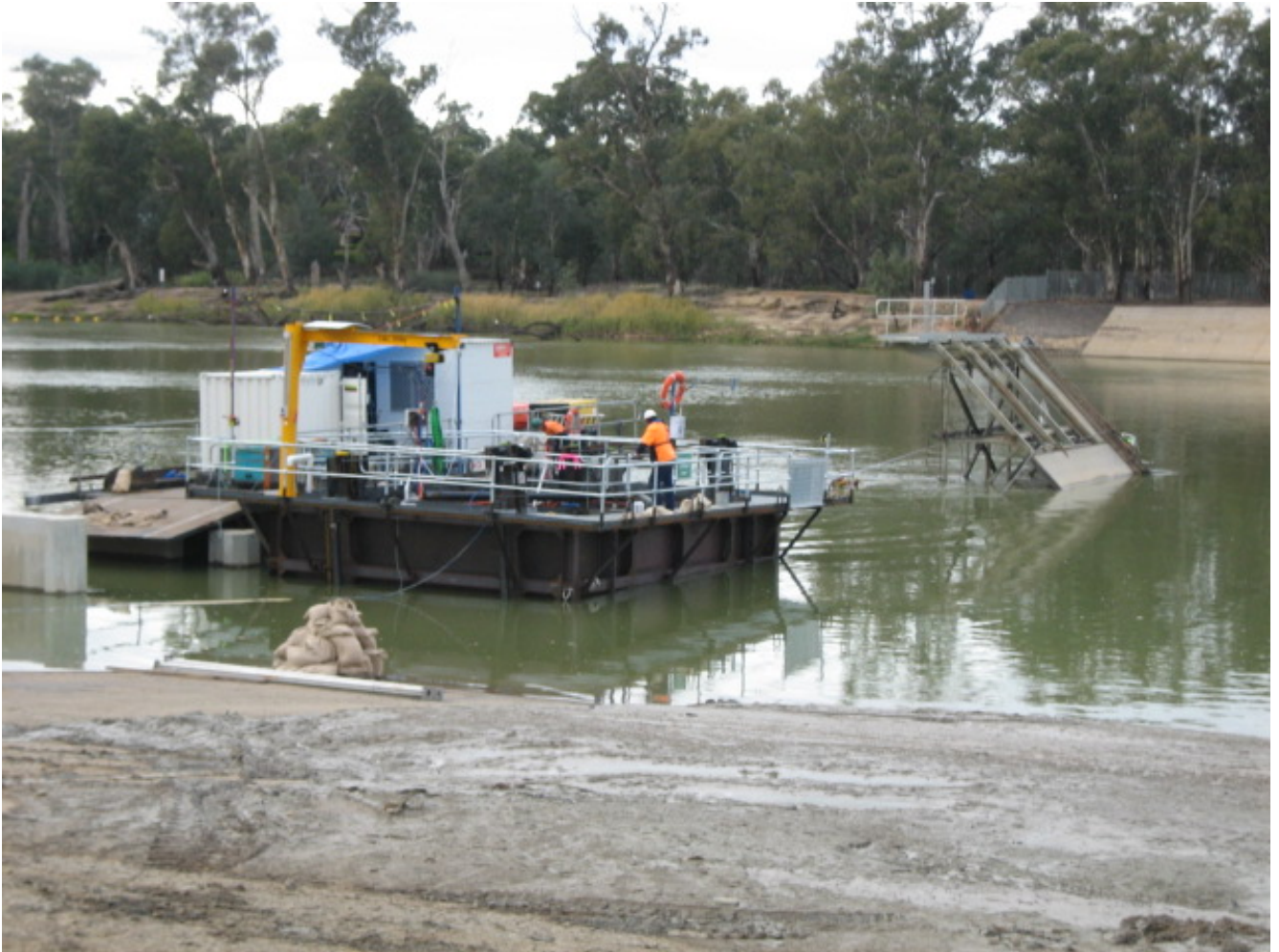
Figure 2 – Works underway at Mildura Weir. Photo supplied by Mathew Fitzgerald, Goulburn-Murray Water.
