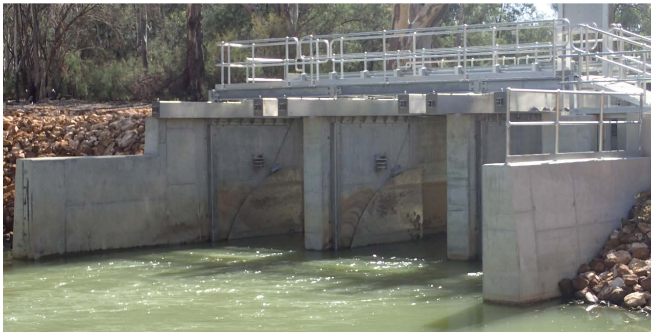
Figure 4 – Mullaroo Creek regulator with all gates lowered. (Photo: SA Water)
