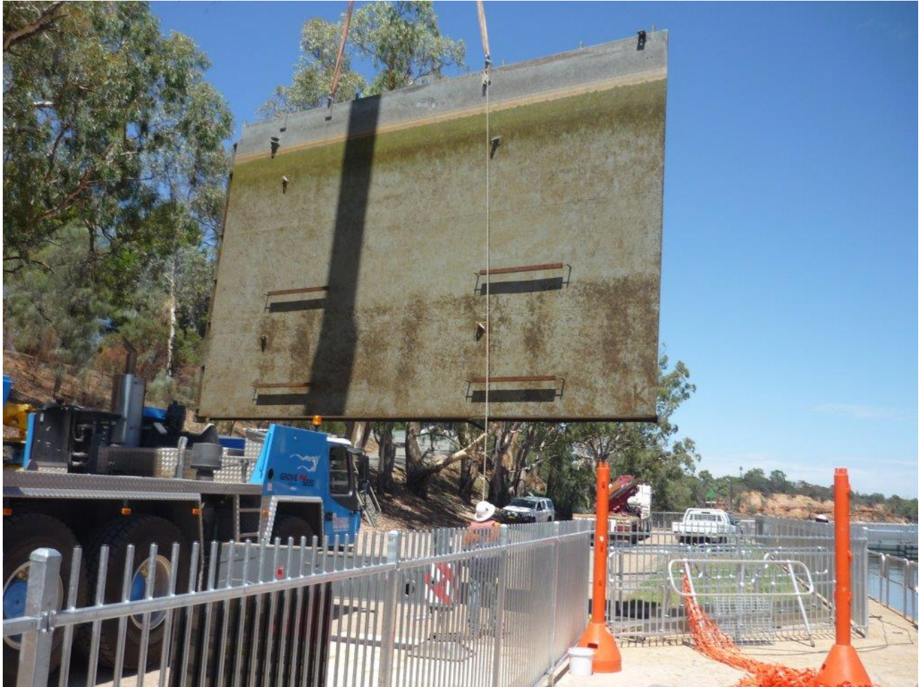
Photo 1 – lifting out the upstream lock gate to repair the hinge bolts (source: Phillip Cocks)
