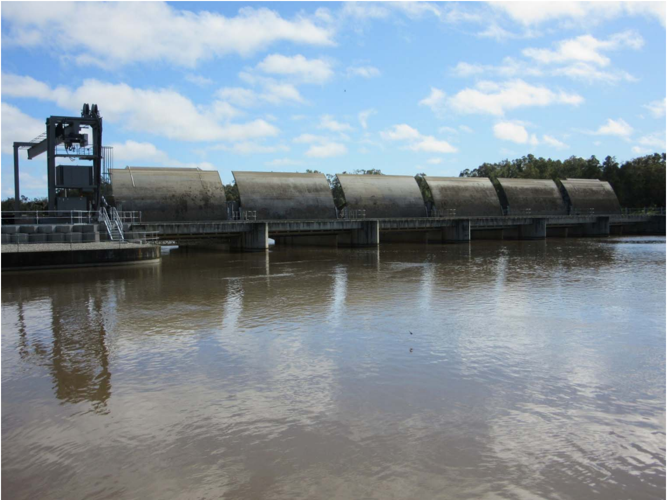
Photo 2- The gates of Torrumbidgee Weir have been lifted clear of the water enabling passage of high flows through the structure (Source: Alana Wilkes, CEWO)
