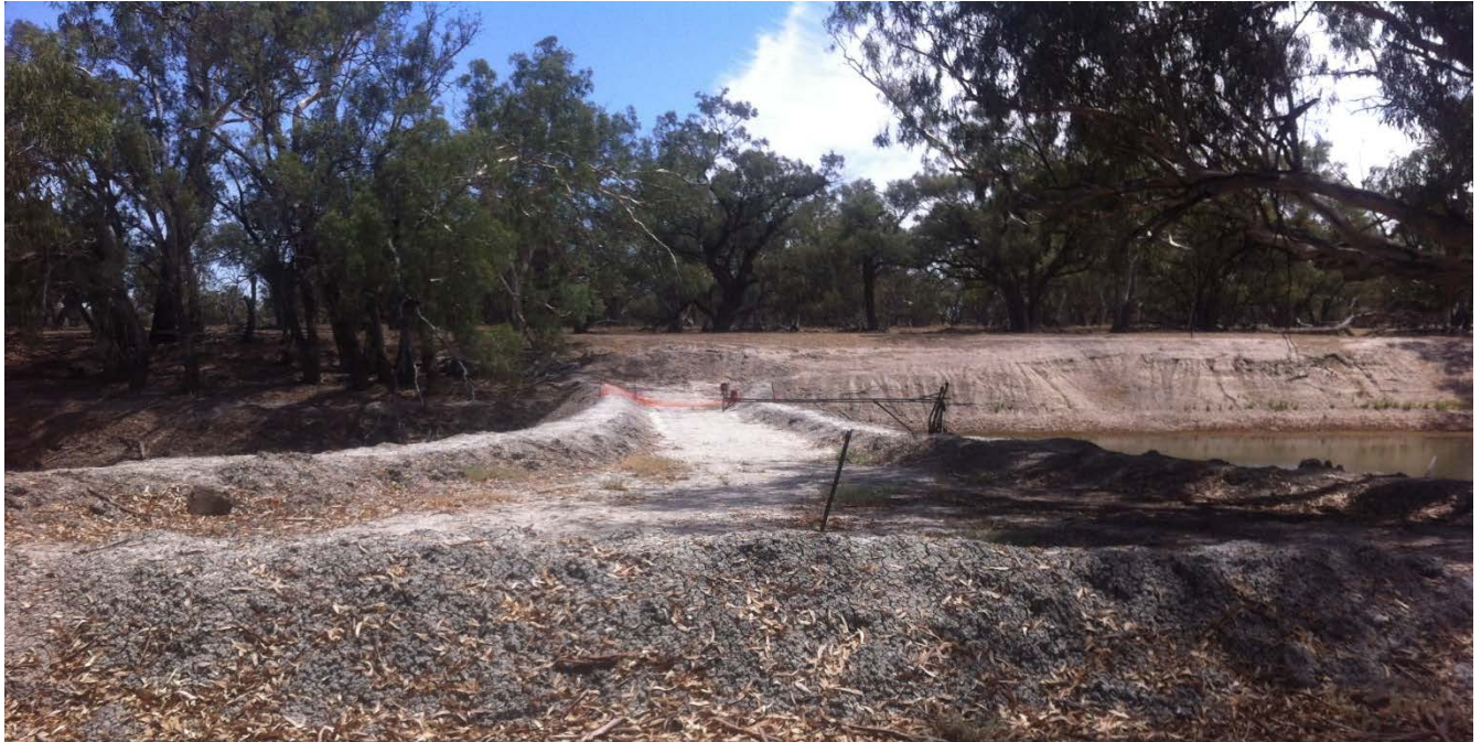
Photo 1 – Installed block bank at Jamesville on the lower Darling River (Source: Jeff Finch, Water NSW)
