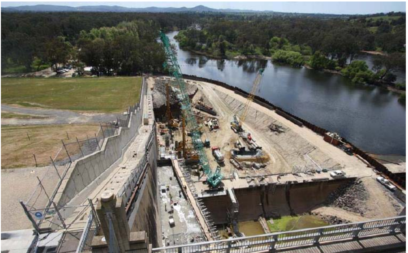
Figure 1 - The southern training wall upgrade construction site at Hume Dam - viewed from the dam wall. The works are taking place directly adjacent to the river downstream. Image: State Water Corporation.
